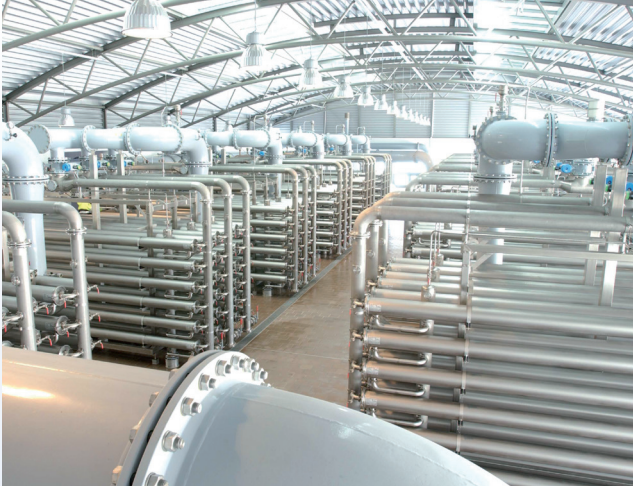
Municipal water treatment facility in Rötgen (Germany)
